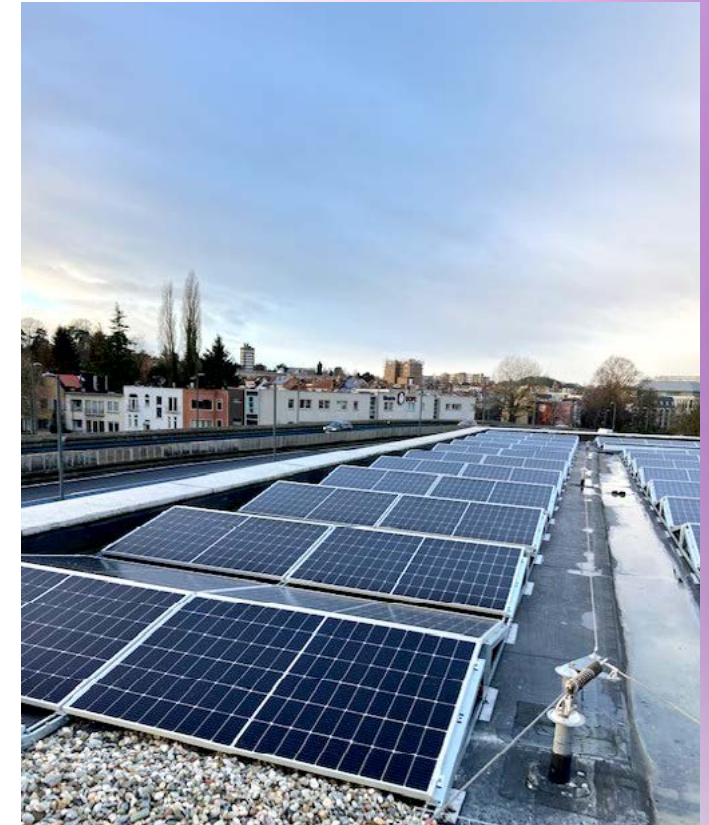
Solar panels on the roof of Marsh McLennan's office space in Belgium.
